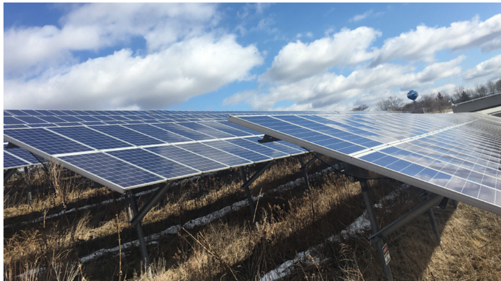
NCRC solar array / Graham Sustainability Institute
